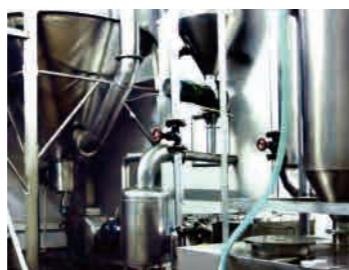
冷冻除湿冷却系统 Desiccant cooling system freezing
